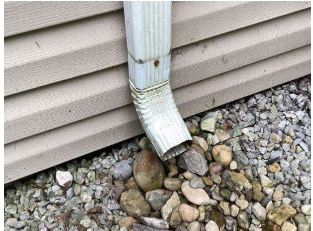
Periodic fastener rust
