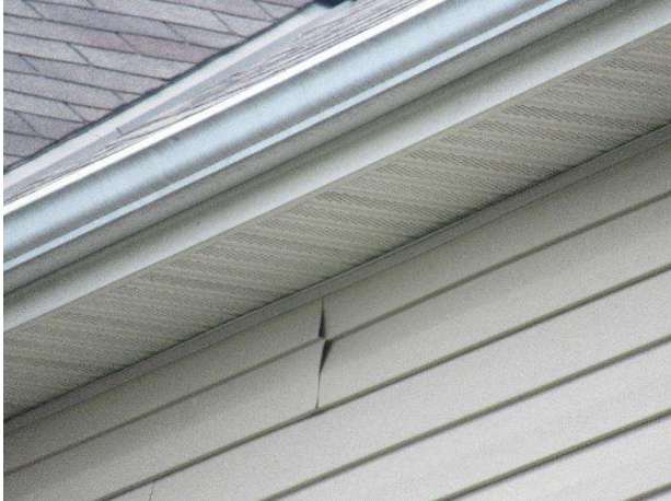
Isolated minor loose siding
