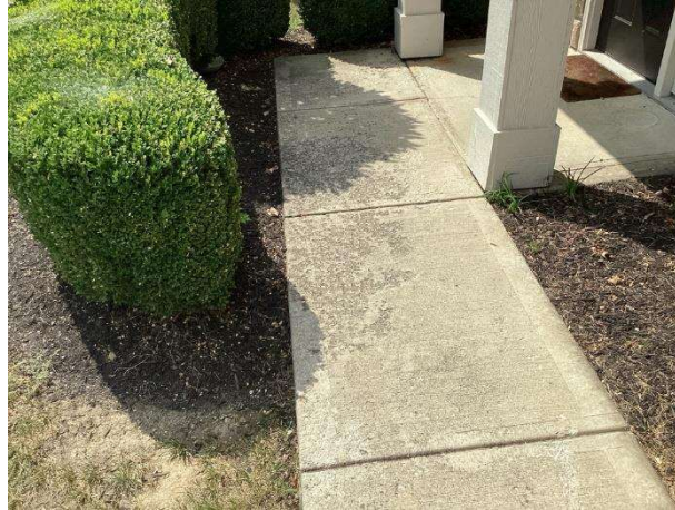
Spall, shown at Unit 9069
