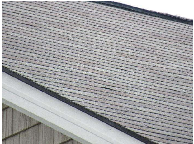
Minor shingle lift, shown at Unit 1439
