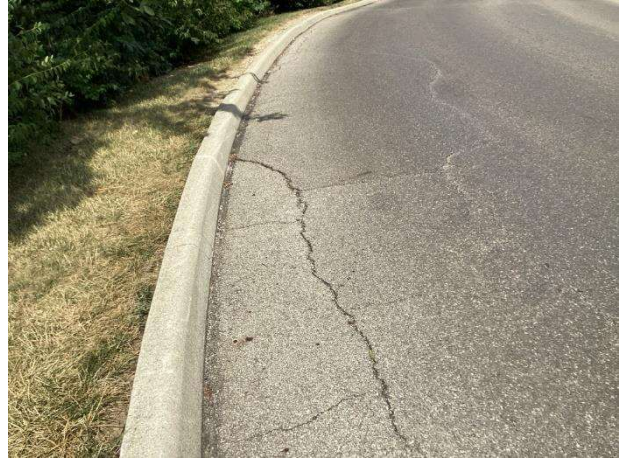
Polaris Lakes Dr settlement cracks (Shared)
