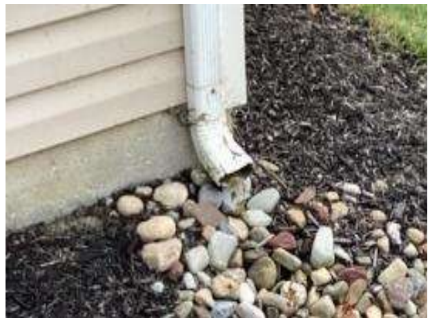
Partially crushed downspout extension
