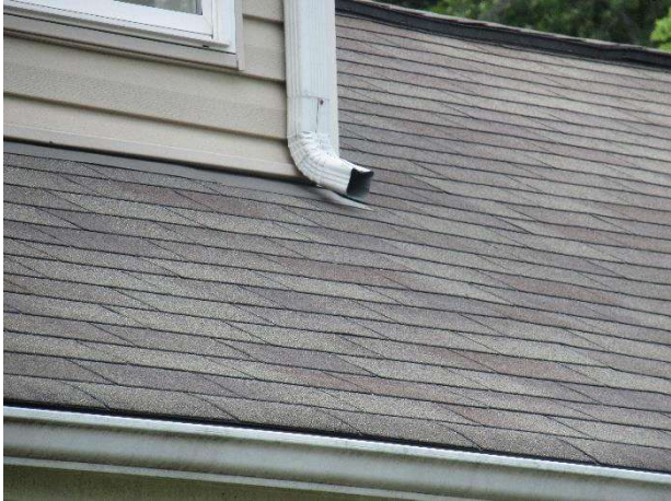
Downspouts discharge onto lower roofs
