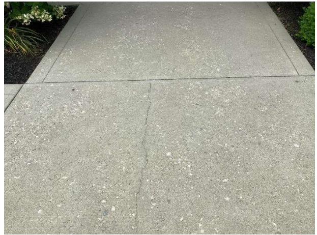
Spall and cracks by clubhouse
