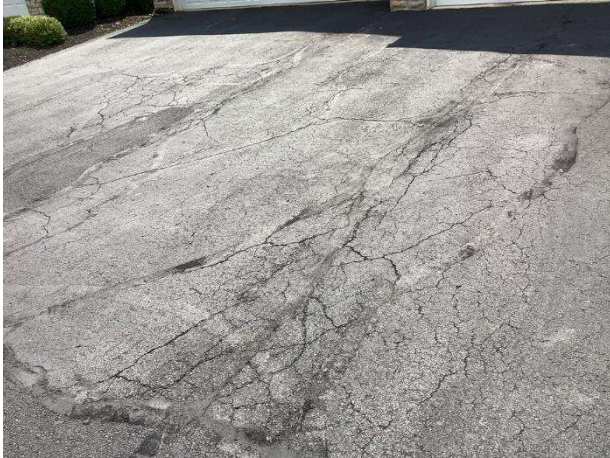
Cracks and deterioration, shown at shared driveway at Units 9109 and 9113
