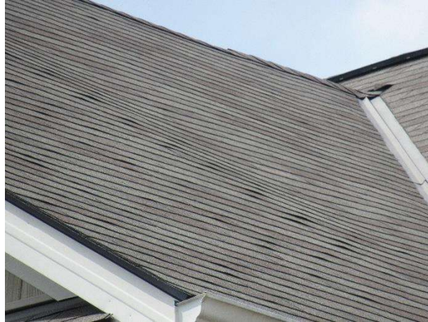
Shingle lift and sheathing deflection, shown at Unit 1420
