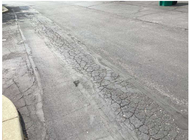
Alligator cracks and previous repairs
