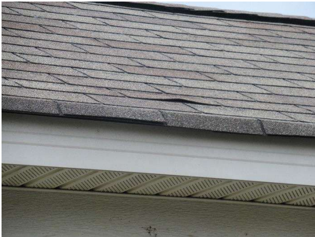
Shingle lift, shown at the mailbox station shelter
