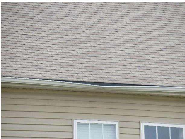
Gutter deflection, shown at Unit 1424
