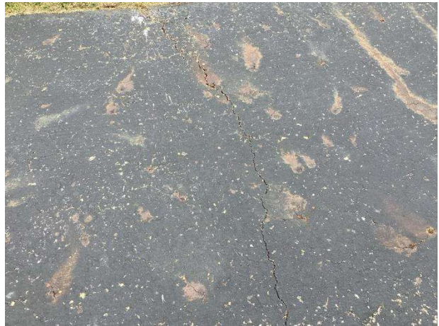
Walking path cracks
