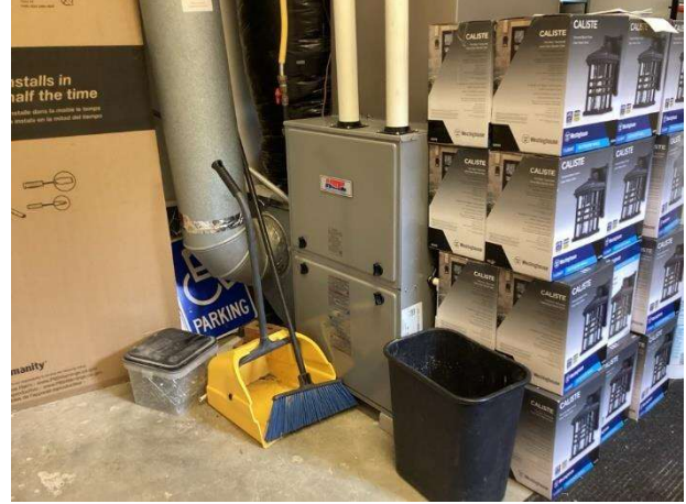
Recently replaced furnace
