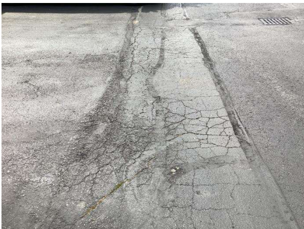
Alligator cracks and surface deterioration
