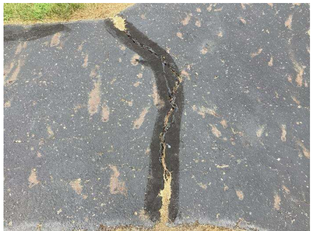
Walking path cracks at previous crack repair
