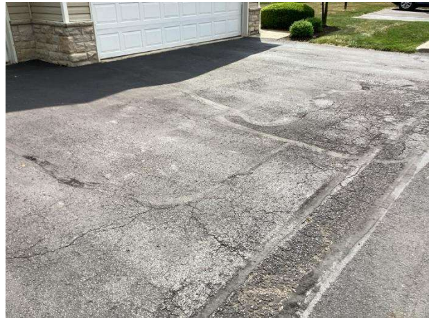
Driveway pavement overview – note deterioration
