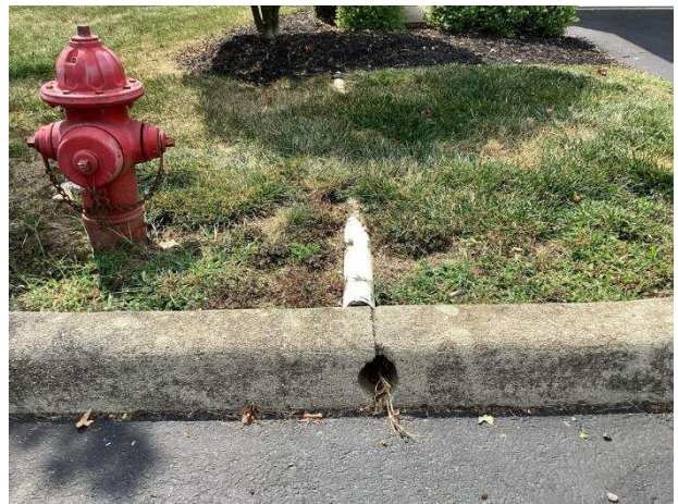
Misaligned drainage pipe, shown by Unit 9065
