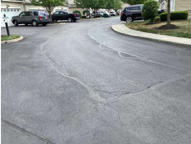
Previous centerline patching
