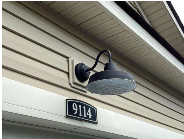
Exterior light fixture at garages
