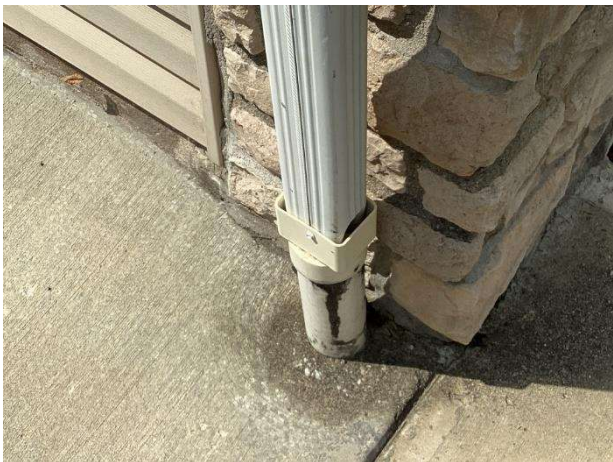
Periodic evidence of overflow at pipe adapters
