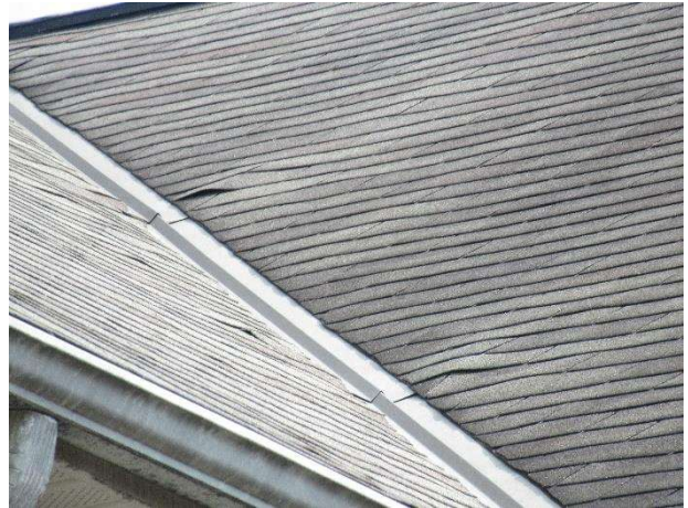
Shingle lift, shown at Unit 9157
