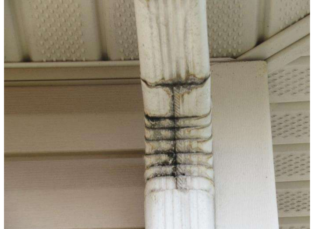
Periodic evidence of leakage at the seams
