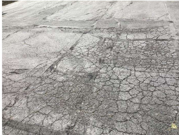
Alligator cracks and surface deterioration
