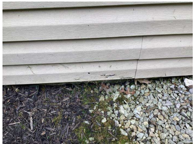
Minor damage, shown at Building 6 rear
