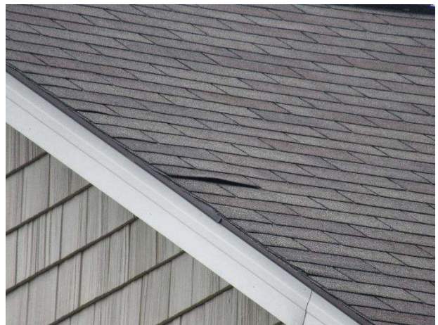
Shingle lift, shown at Unit 9128
