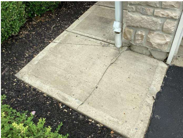
Concrete damage, shown at Unit 9153
