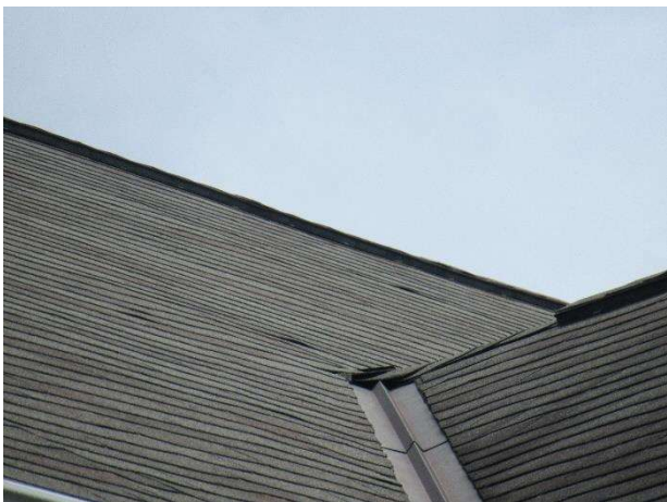
Periodic shingle lift
