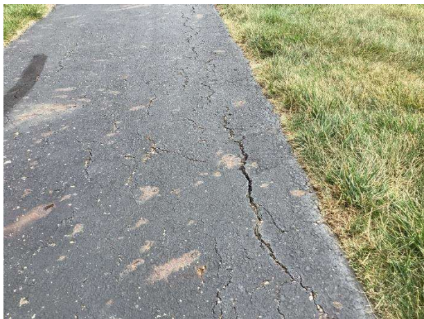
Walking path cracks
