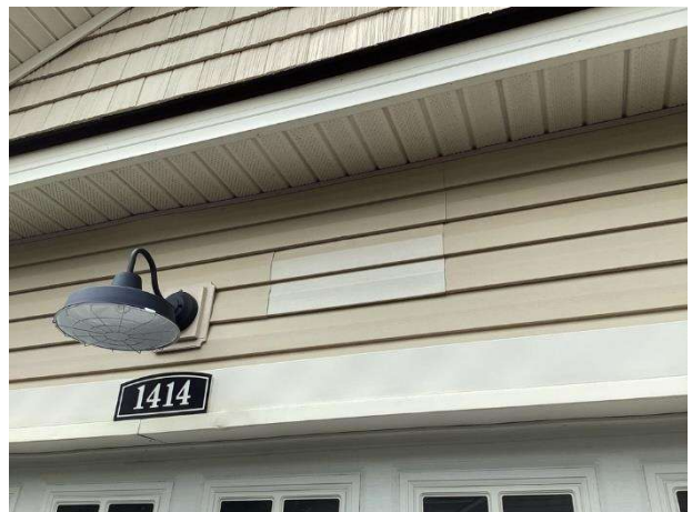
Non-uniform previous partial replacement, shown at Unit 1414
