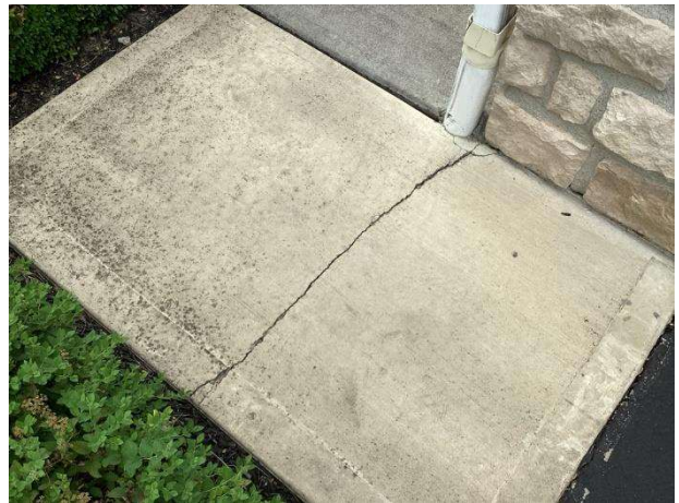
Concrete damage, shown at Unit 9148
