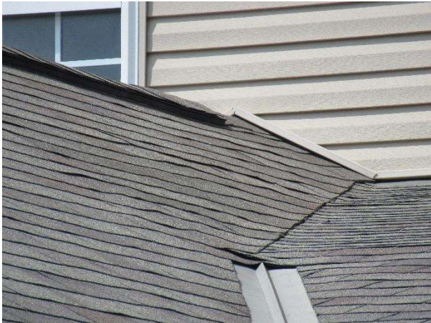
Shingle lift, shown at Unit 9178
