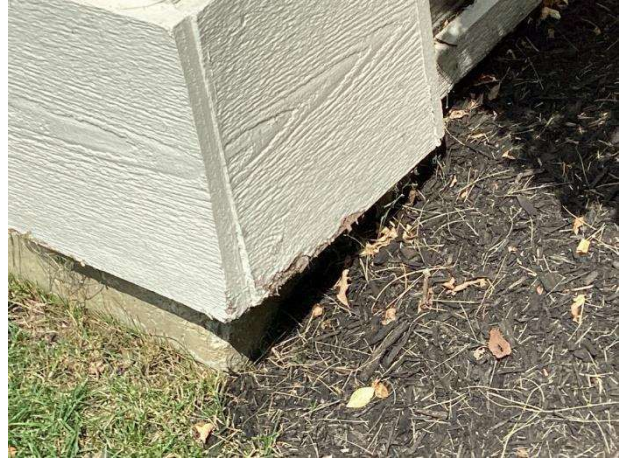
Minor finish deterioration
