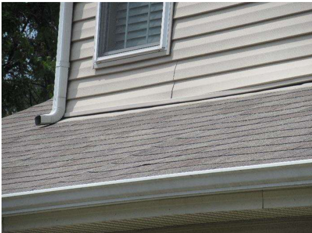
Sheathing deflection, shown at Unit 9020
