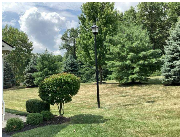
Light pole and fixture
