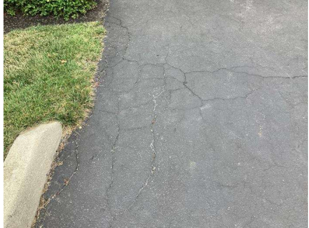
Alligator cracks, shown at Unit 9148
