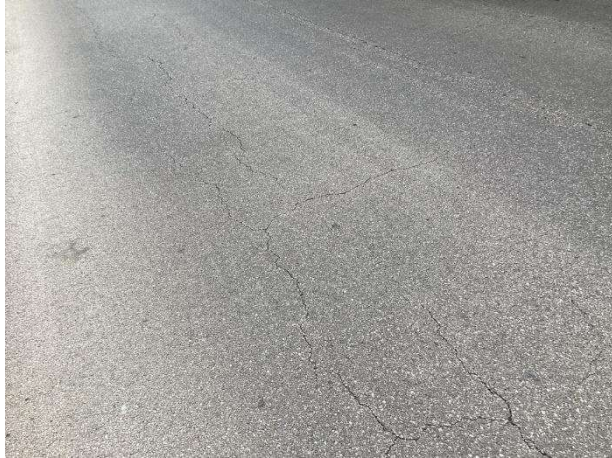
Polaris Lakes Dr pavement cracks (Shared)
