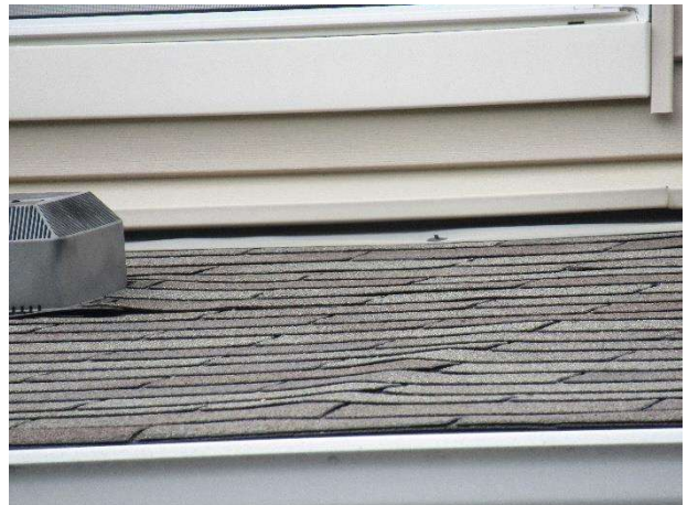
Sheathing deflection, shown at Unit 1450
