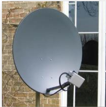
Satellite Dish - Ground Mounted
